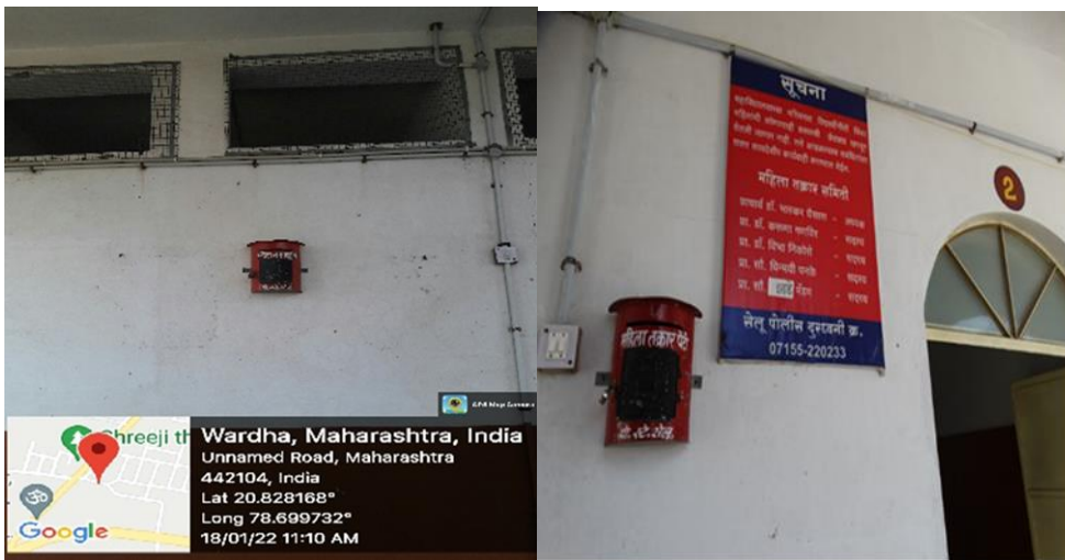
In college campus there is a complaint box (Mahila Takrar Peti) installed in corridor.
