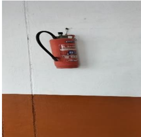
Fire extinguisher for safety
